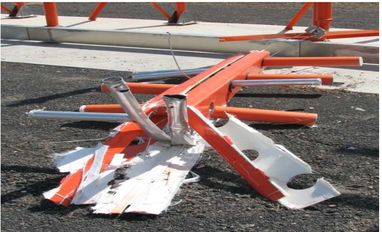
Damaged localiser antennae
